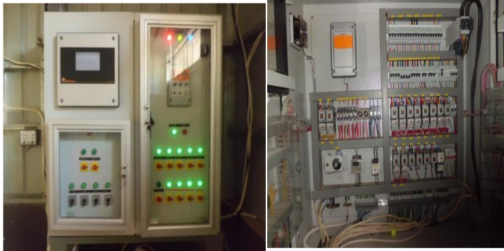
Gambar 11. Panel Outomatic Controlling
