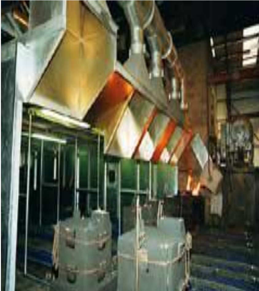
Fume extractor system
